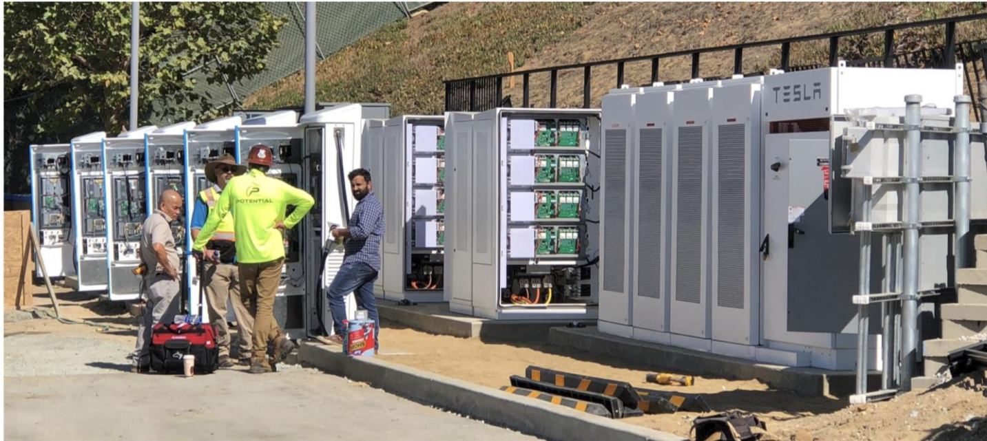
Single & dual output dispensers | 480 VAC/DC conv. cabinets | 480V AC switchgear & 4 battery Powerpacks
